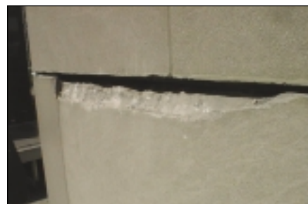
Stone observed after a loose spall has fallen to the ground.
