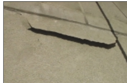
Loose spall in stone (removed during inspection for safety).
