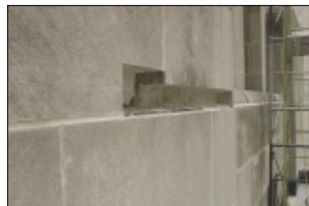
Spalled stones are cut and ready to receive dutchman repairs. The process involves replacing a small portion of the stone with new stones cut to fit and then mortared into place.
